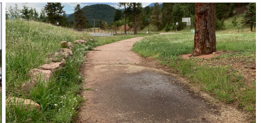
8 ADT in need of repair and dog waste stations.
