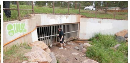
7 Fountain Creek culvert is an attractive nuisance.
