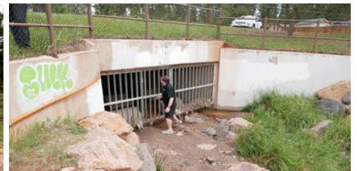
7 Fountain Creek culvert is an attractive nuisance.
