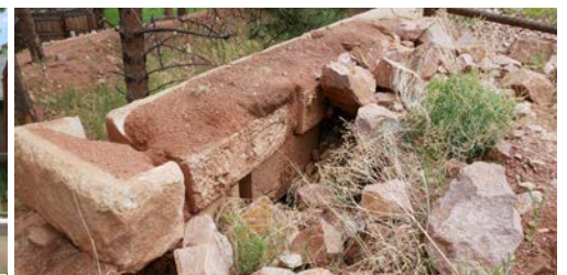
4 Drainage issue and compromised retaining wall.
